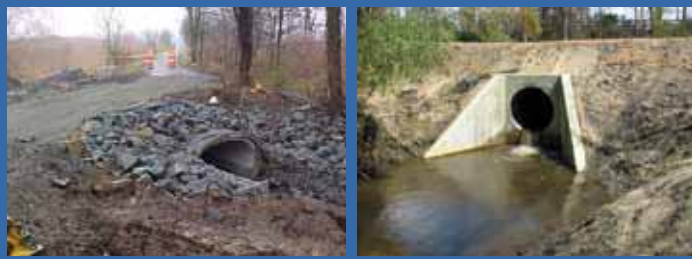
Besides bridges, another major construction project when converting railways are rehabilitating the culverts, shown here for the HHT (left in 2002) and UTT (right in 2009).
