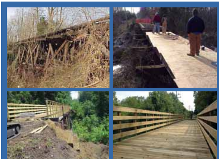
These photos of the trestle bridge rehabilitation over Lahaway Creek hint at the trail's past use as a railroad.
