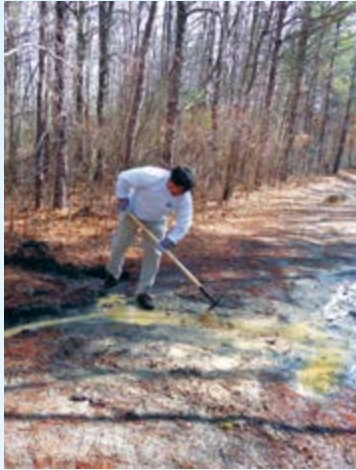
Volunteer Al Fico digs a winding trench into the woods to route water off the trail.
