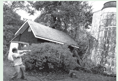
Ray Smith, a Carpenter with Construction and Repair, holds up this leaning silo in the Claypit Creek section of Hartshorne Woods so it can be stabilized. This silo (manufactured in the early 20th century) along with other structures nearby, hint at the presence of a small scale, "gentleman's farm" operation at this site. The silo probably stored corn silage used as animal feed for cows.
