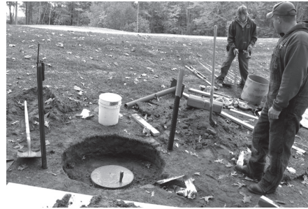
C & R Electrician Dave Hollabaugh (left) and Charleston Springs Senior Greenskeeper Mark Foulks (right) install the cement base for one of the fans, last fall.
