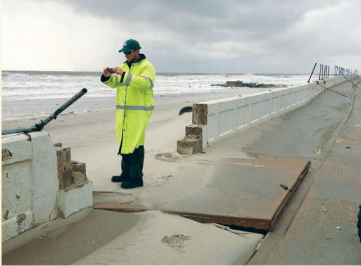
Under a still-angry sky the day after the storm, Seven Presidents Oceanfront Park Manager Ryan Rochelle starts to assess damage to the 'sea wall' on the north end of the park.
