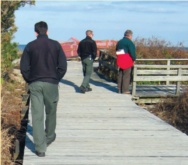
(l to r) Park Managers Matt Coleman and Ryan Rochelle assess boardwalk damage with Senior Engineer Jim Mowczan of A&D.
